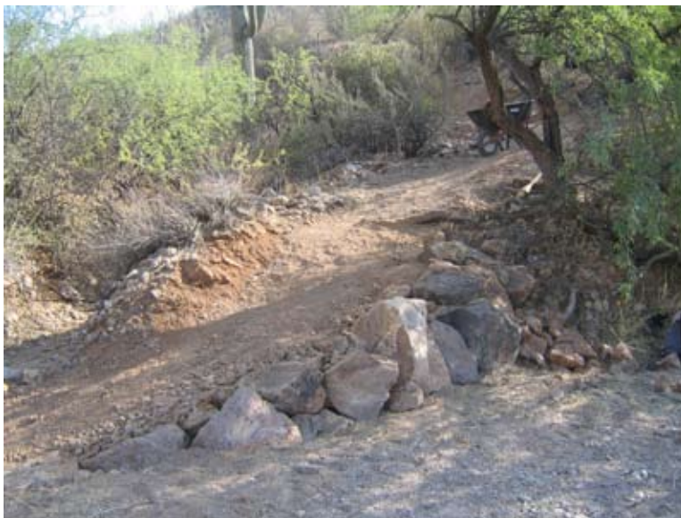
The large rocks in this crib wall, which supports a trail as it enters a junction between a large wash and a side wash, protect the trail when the wash is running.
