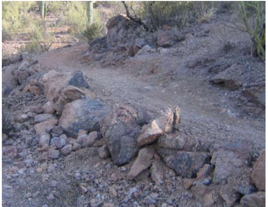
This crib wall raises the trail above bedrock, providing a nice, even tread.
